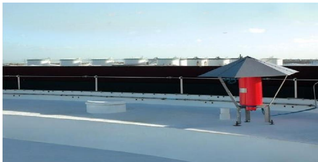
Figure 10: Rim Seal Fire Protection System
