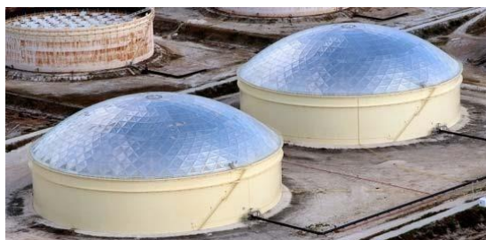
Figure 9: Geodesic roof tank
