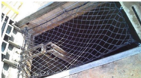
Figure 5.6 Use of safety nets
