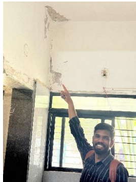
Fig.2 Flaking of Paint & Plaster
