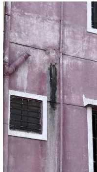
Fig.1 show the dampness present in the building structure.
