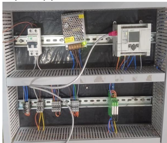
Fig.-3 PLC Setup
