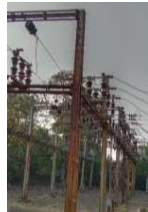
33kV Bus Structure
